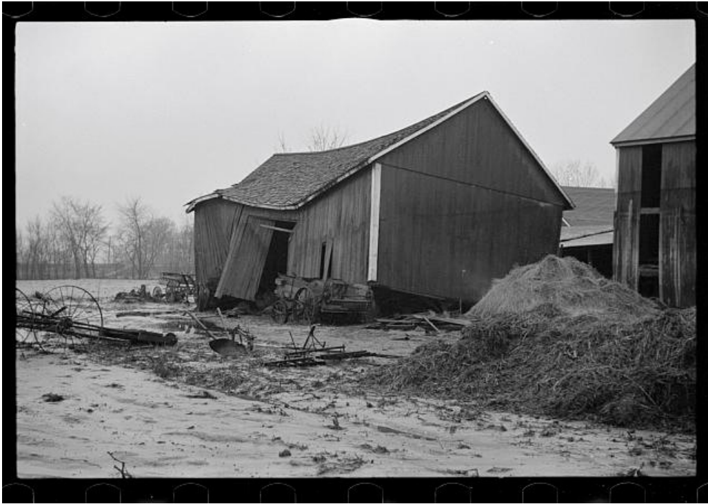
Figure 4: Barn damage from the 1936 flood
